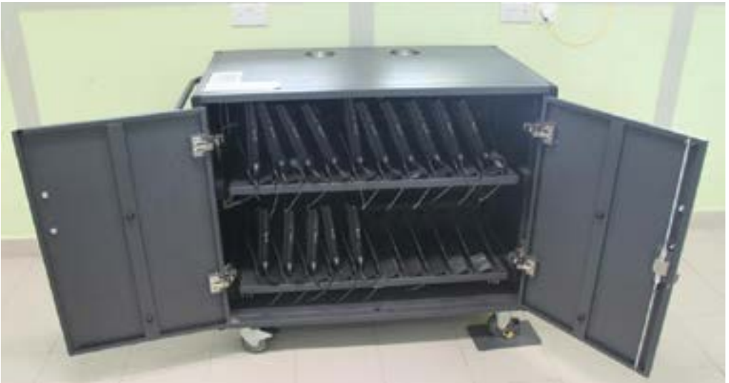
Figure 2.8 Mobile storage cart for storage and charging of the notebook computers in the classrooms
